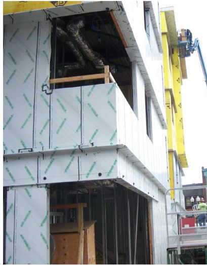
Air barrier installation around openings and projections. Photo courtesy of Len Anastasi
